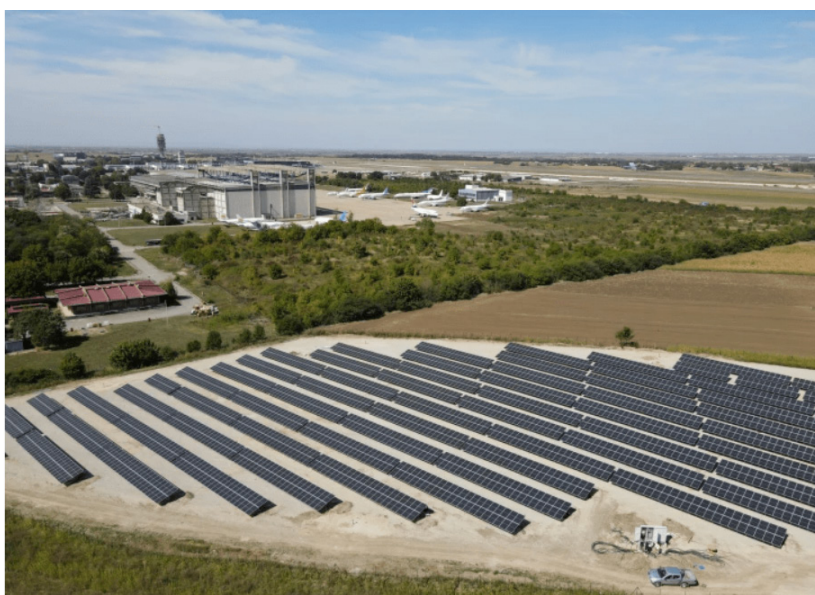
Figure 12 Solar Plant – Courtesy of Vinci Airports
