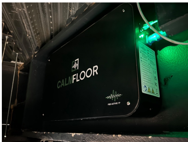
Figure 3: The 67kg CALMFLOOR AMD attached to a steel I-beam supporting a composite steel-concrete deck. Courtesy of FSD Active Ltd.
