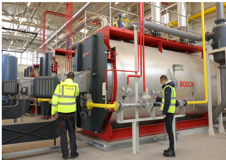
Figure 11 Heating Plant – Courtesy of Vinci Airports
